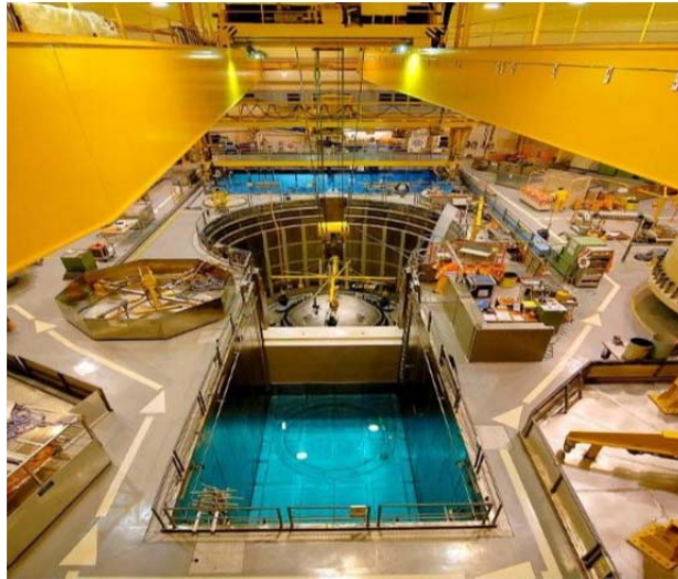
Figure 1: Refuel floor of a reactor.
